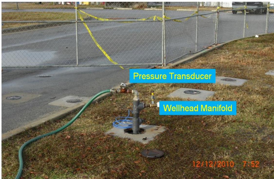
Figure 5-16. Injection wellhead manifold and pressure monitoring.
